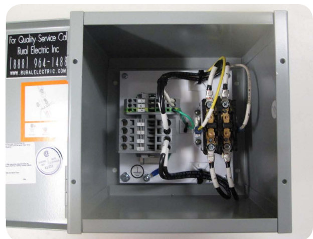
Heliport Control Box
